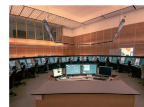
Installed monitors in Belgocontrol's Tower and aviation center in Belgium
